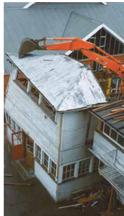
1983 - demolition of the end rooms of Erwin - the Junior House which was added in 1925.
